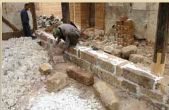
Reinstatement of stone foundation and repair of timber structural post. (Shaxi, Yunnan 雲南沙溪興教寺)
